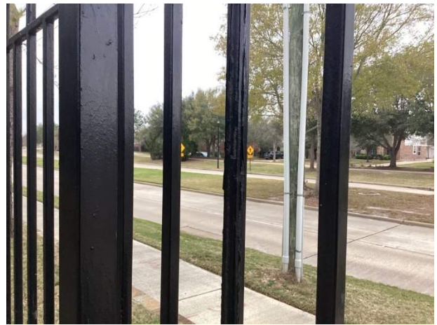
Fence finish deterioration
