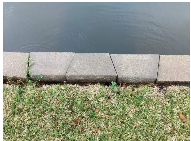
Masonry displacement at the villas
