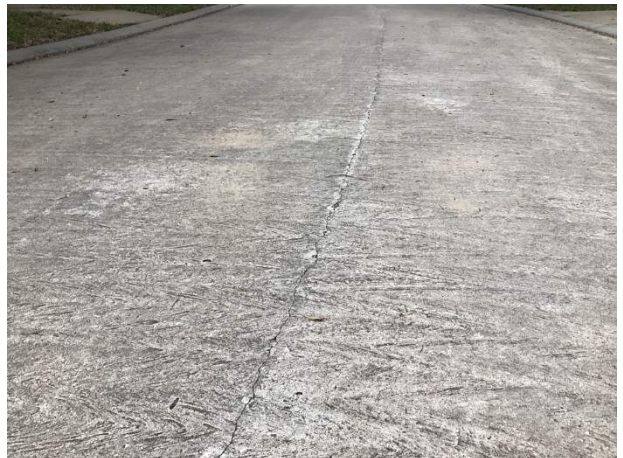
Centerline cracking at the Lakes
