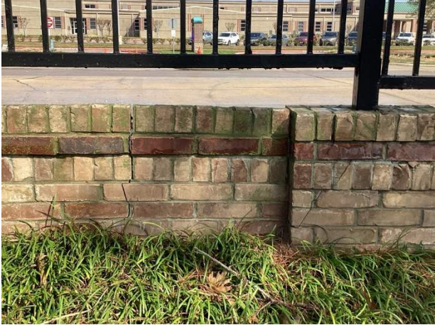
Wall cracks at the manors
