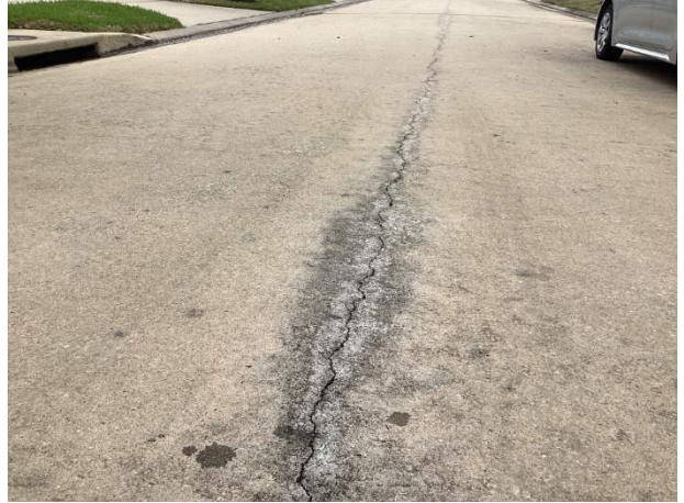
Street cracks at the Estates
