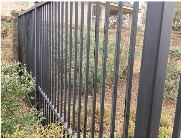
Fence finish deterioration at the lakes
