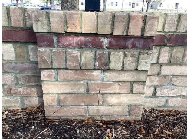
Wall cracks at the manors
