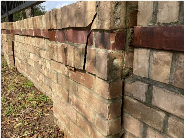
Wall cracks at the manors
