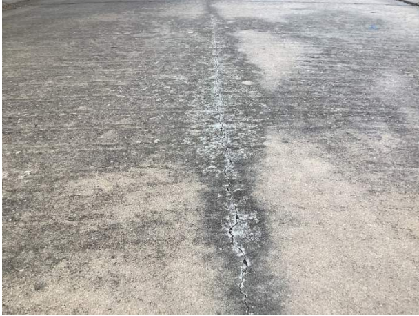
Centerline cracking at Lakes West
