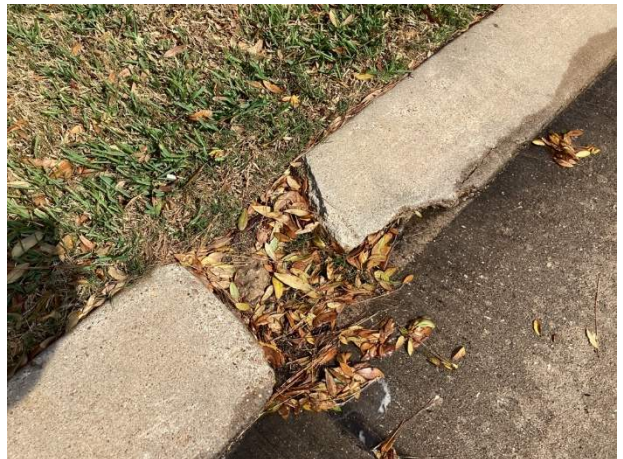
Concrete curb spalling at the Manors
