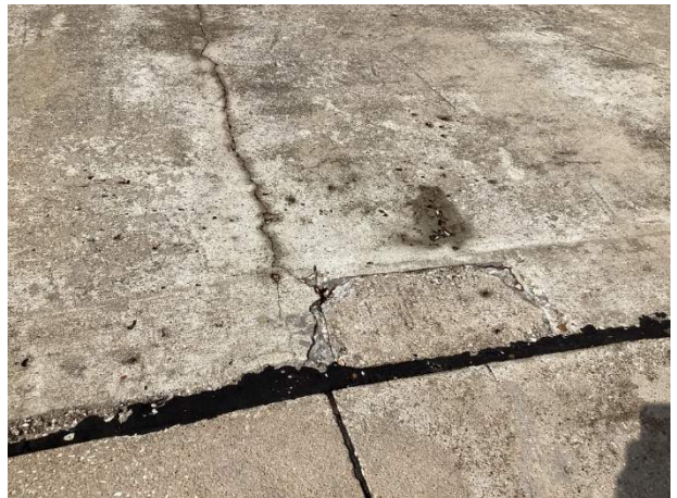
Street spalls at the Villas
