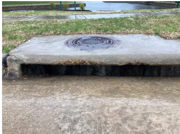
Concrete deterioration at Lakes West
