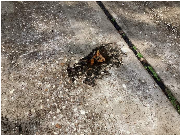
Street spalls at the Villas
