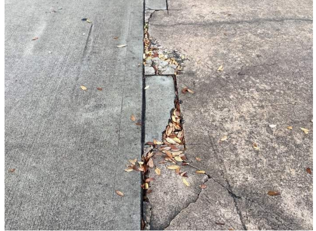
Street spalls at the Villas
