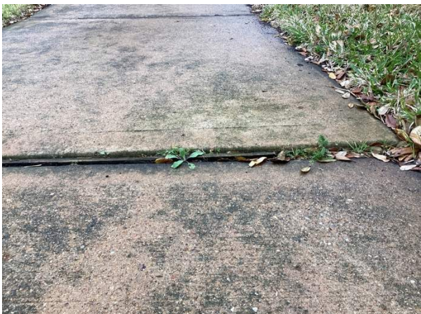
Sidewalk trip hazard
