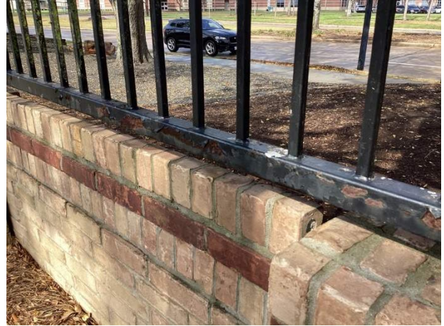
Fence rust at the manors
