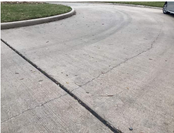
Street cracks at the Lakes
