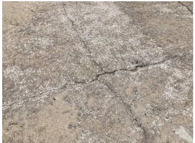
Street cracks at the Estates
