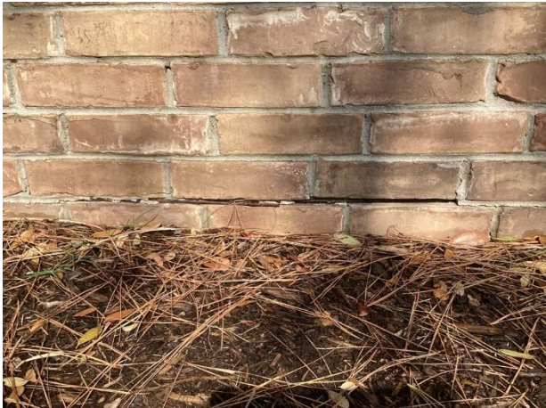
Wall exposed support wire at the manors
