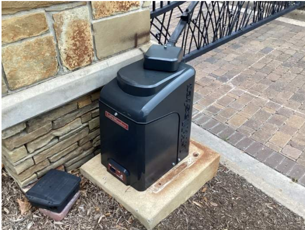
Gate operator at the villas
