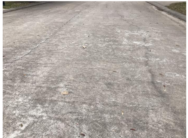
Street cracks at the Lakes
