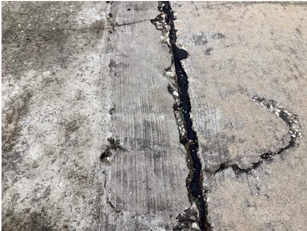
Street spalls at the Villas
