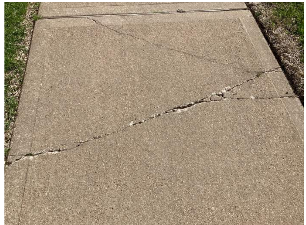
Sidewalk cracks at the Villas
