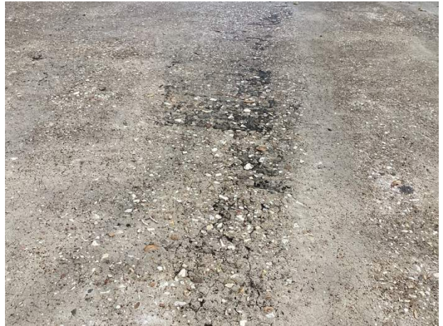
Street deterioration at the Villas
