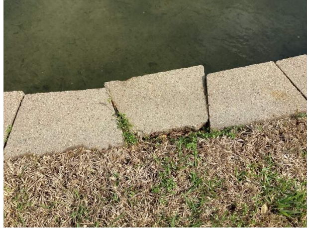
Masonry displacement at bulkhead
