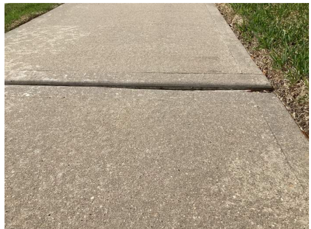
Sidewalk trip hazard
