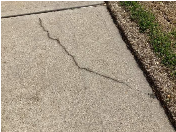
Sidewalk cracks at the Villas
