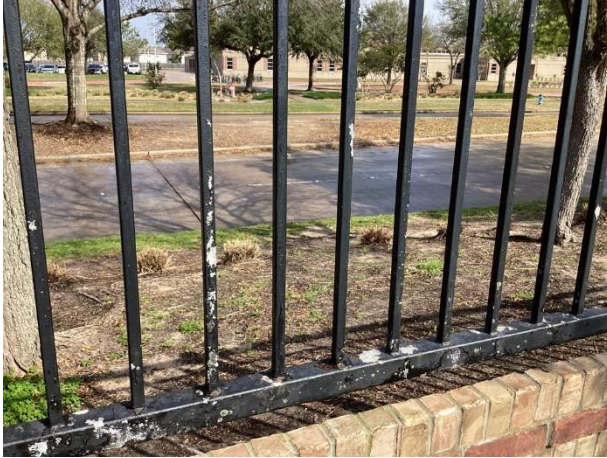
Fence finish deterioration at the manors
