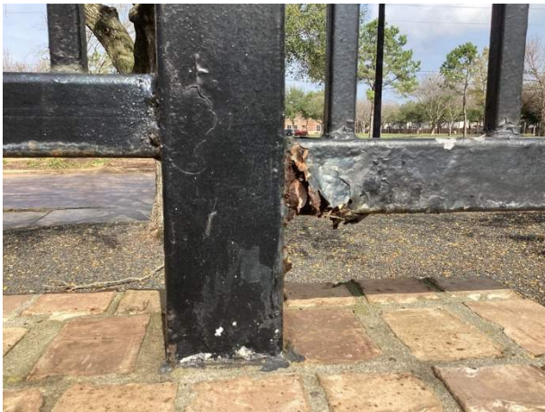
Fence rust at the manors
