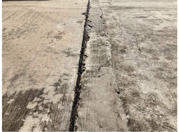
Street deterioration at the Villas
