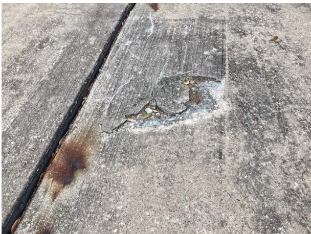
Street spalls at the Lakes
