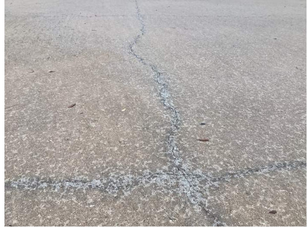
Street cracks at Lakes West
