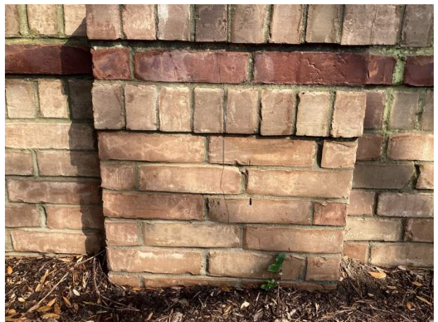
Wall cracks at the manors
