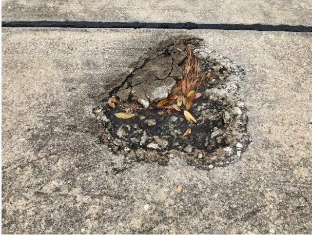
Street spalls at the Estates
