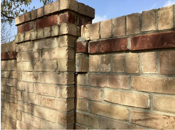
Dislodged masonry at the manors
