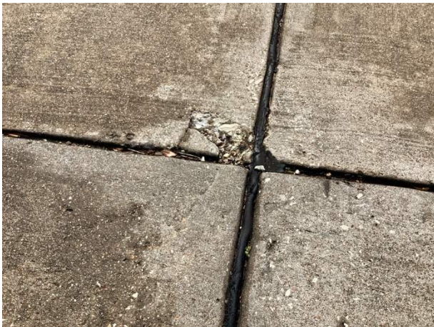
Street spalls at the Manors
