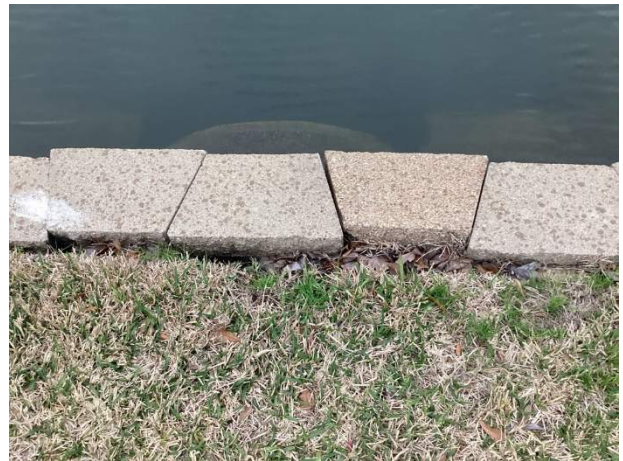
Wall displacement at lakes west
