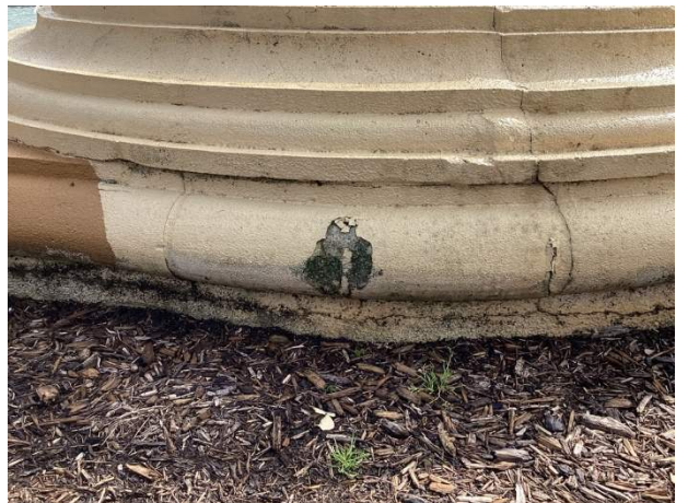
Paint finish deterioration
