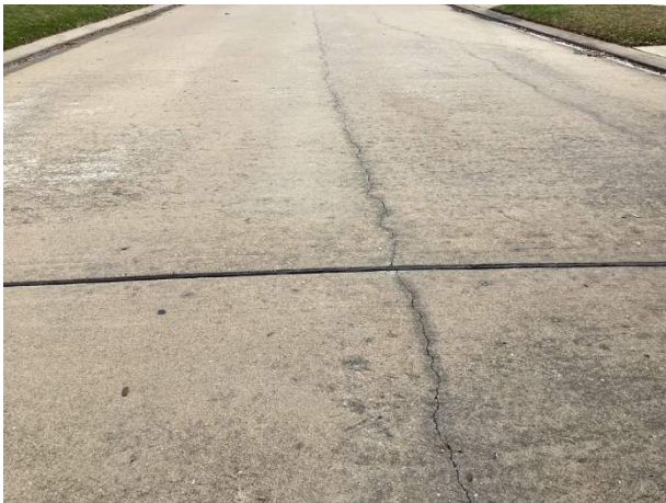
Street cracks at the Estates
