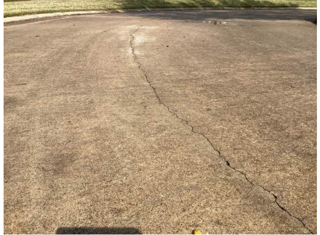
Street cracks at the Manors
