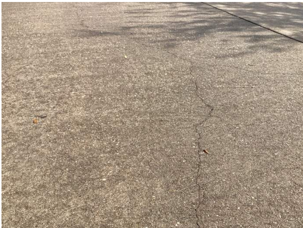
Street cracks at the Manors
