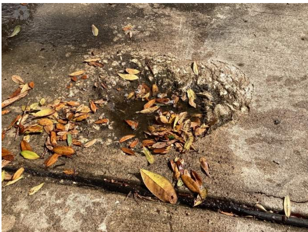
Street spalls at the Villas
