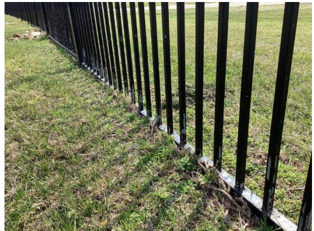
Fence finish deterioration at the villas
