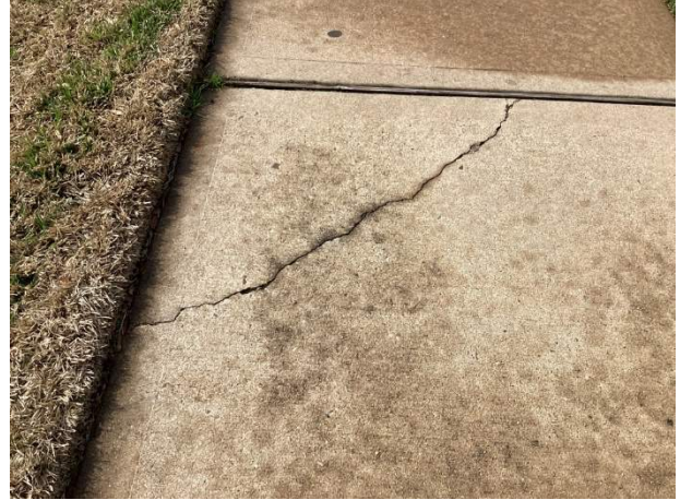
Sidewalk cracks at the villas
