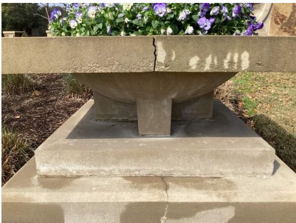
Masonry cracked at front entrance planters
