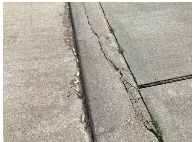
concrete curb cracks at the Villas
