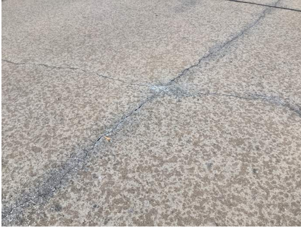
Street cracks at Lakes West
