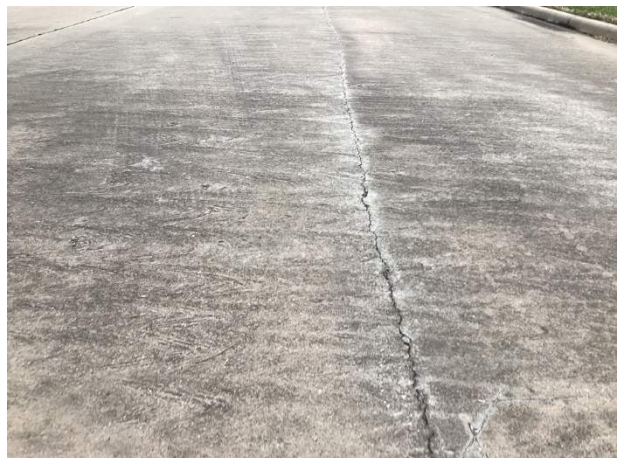
Street cracks at the Lakes
