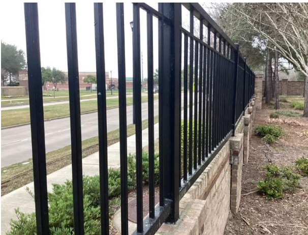
Steel fence at the lakes
