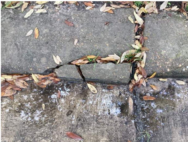
Concrete curb cracks at the Villas
