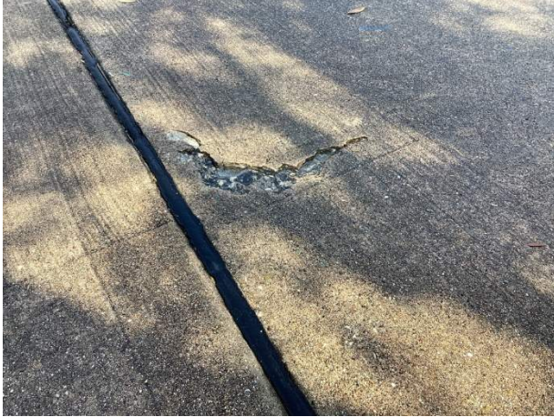
Street spalls at the Manors
