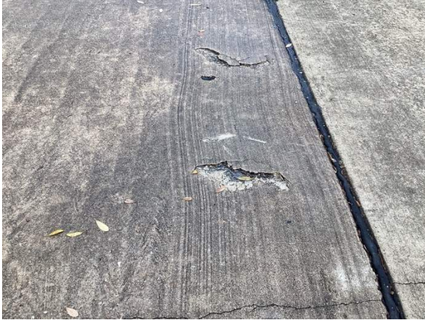
Street spalls at the Villas
